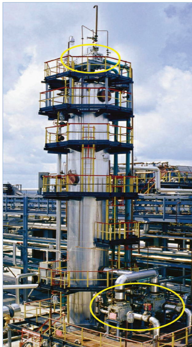
Figure 3. Stripper tower at Yukos refinery. The Compabloc reflux condenser and reboilers are highlighted.
