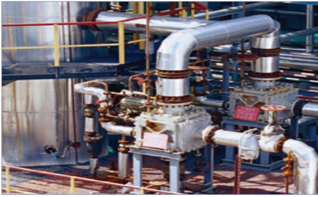
Figure 4. Compabloc thermosiphon reboilers at Yukos refinery working with steam as heating media.
